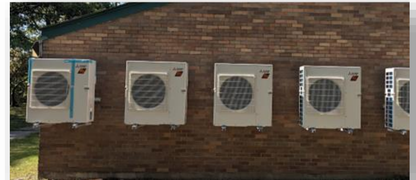
This is a photo of an electrification and solar + battery project at LDF.
